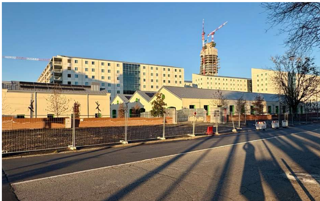
Fig. 4. The construction site of the Athletes' Village at Porta Romana in December 2025, two months prior to the opening of the Games. Source: Authors
